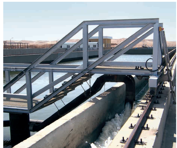
Return sludge channel with pressure pipes
